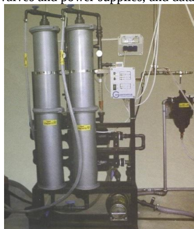
Fig. 2: Ion-exchange columns combined with automatic self-cleaning mechanical filters (modules 5 and 6)
