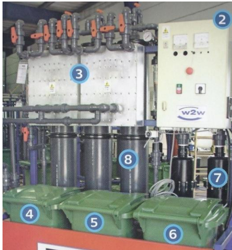
Fig. 3: Water treatment and regeneration system with electrochemical reactors and filtration modules
