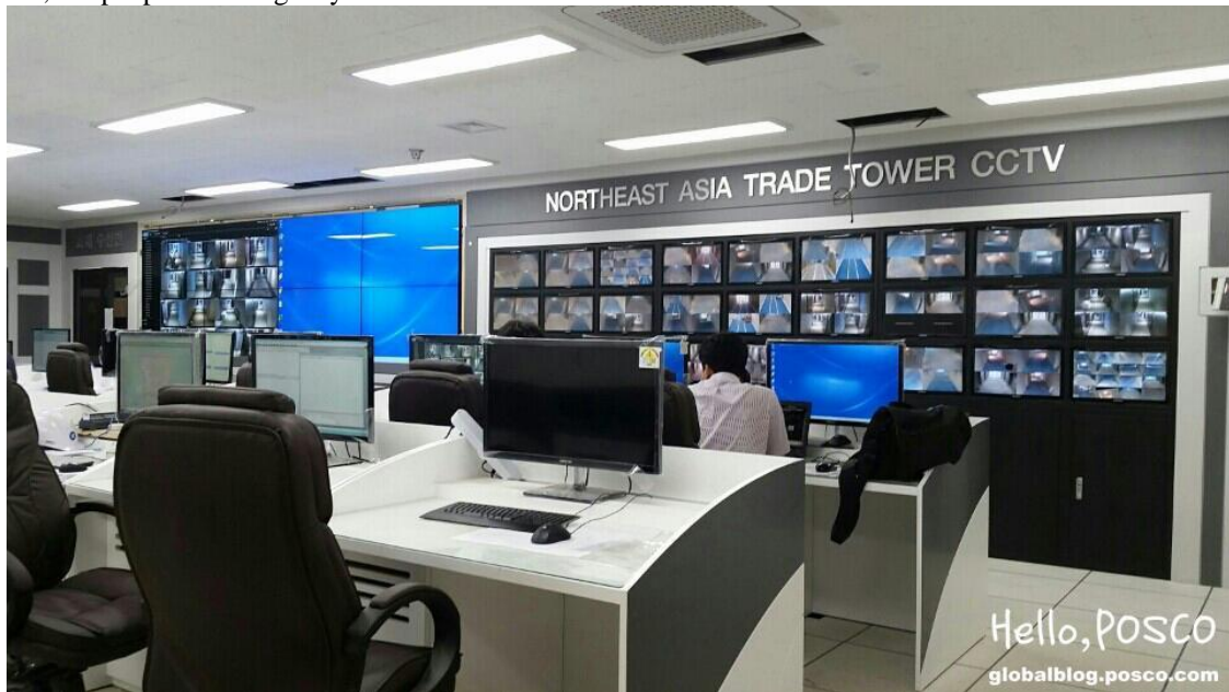
Fig. 8: Emergency control centre located on the basement floor
