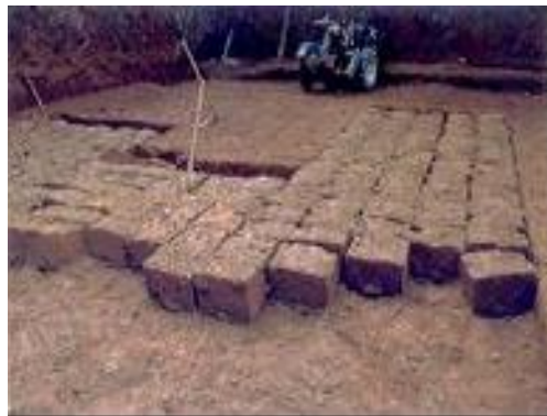
Fig. 1 Machine quarrying of laterite masonry blocks (a) Quarrying of laterite using mobile rotary saw machine; (b) Laterite blocks detached from the bed
